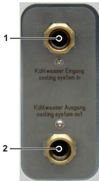
Fig. 18: Connections for the water cooling system
